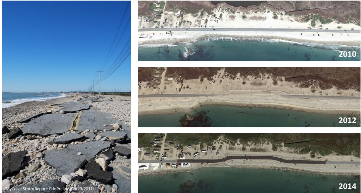
Figure 9 East Beach Road damage from Hurricane Irene.
