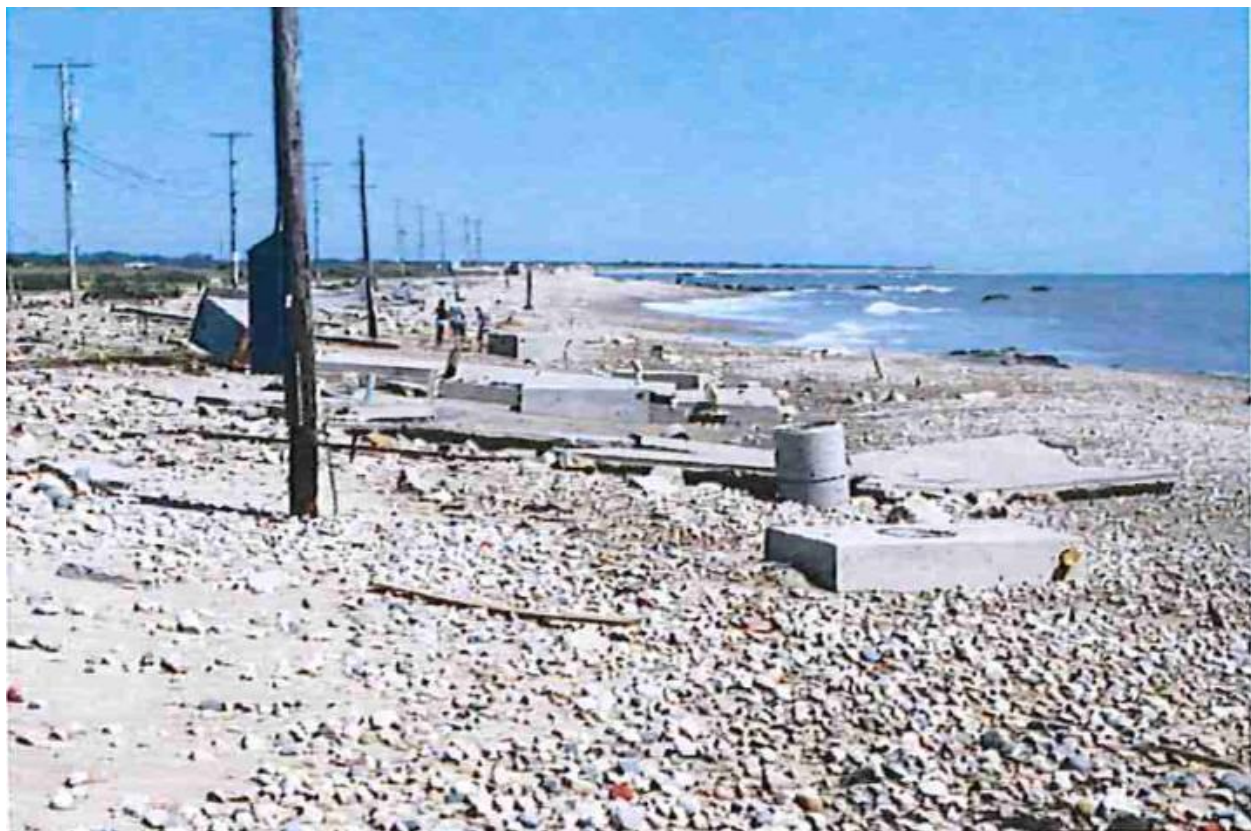
Figure 10 Exposed and damaged septic tight tanks on East Beach after Hurricane Irene.
