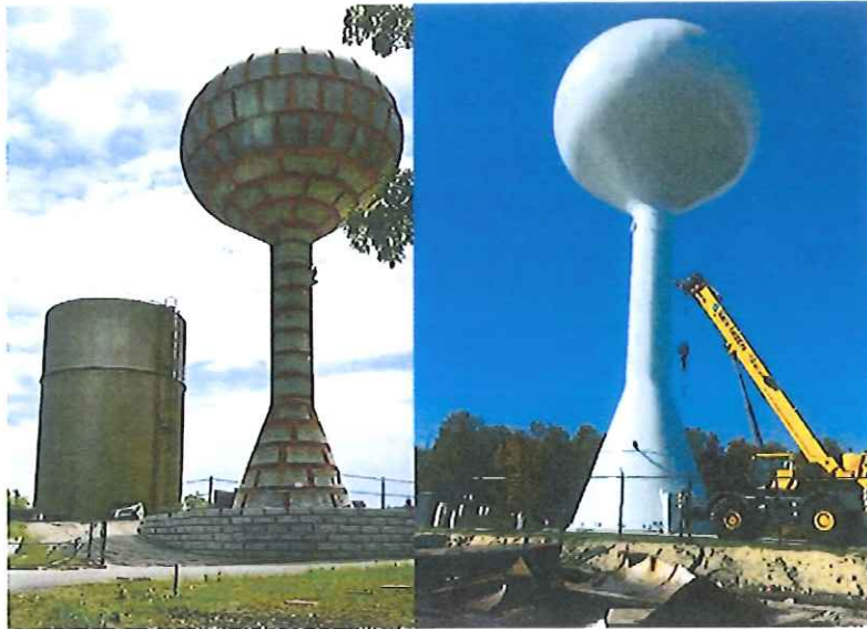
Shown above: Partly completed new airport Rd. elevated tank with old tank alongside (left), and new tank almost complete (right)
