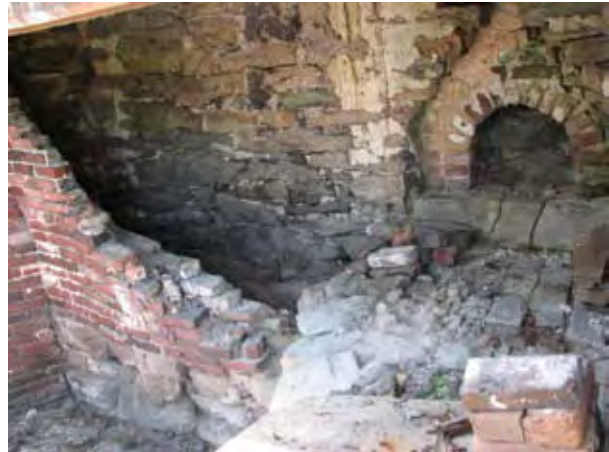
Figure 5.4: The opening for the original bake oven behind the later brick firebox insert in the east hearth.
