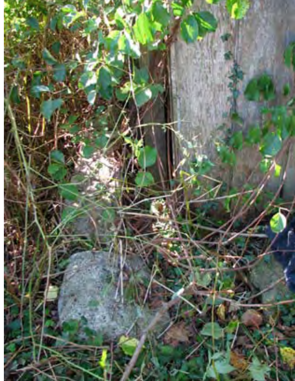
Figure 4.11: Foundation stones for previous shed just outside the northwest corner of the modern shed.
