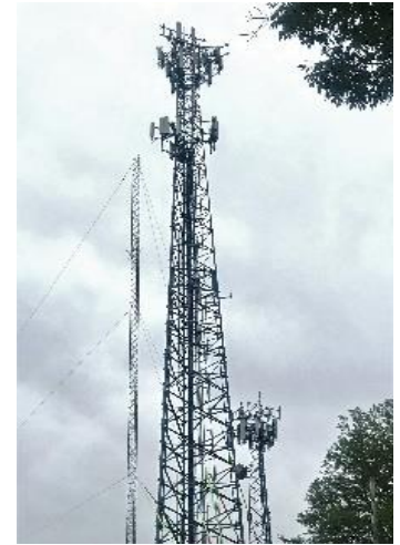
MAIN ROAD CELL TOWER
